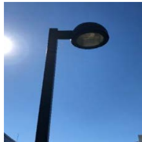
Pole Mounted Parking Lot Lighting
