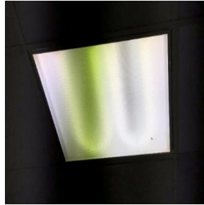
U-Bend Fluorescent Lamp Fixture
