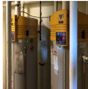
DHW Heaters near Locker Rooms
