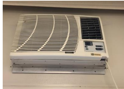
Window AC Unit
