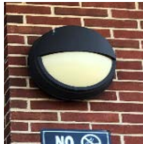
Wall Mounted Fixture
