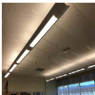
Classroom Lighting Fixtures
