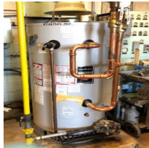
DHW Heater in Mechanical Room
