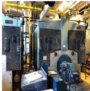
Hot Water Boilers
