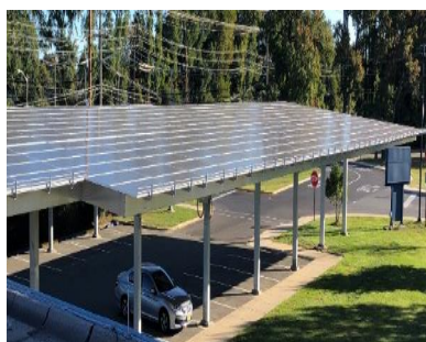
Solar Array Above Parking Lot
